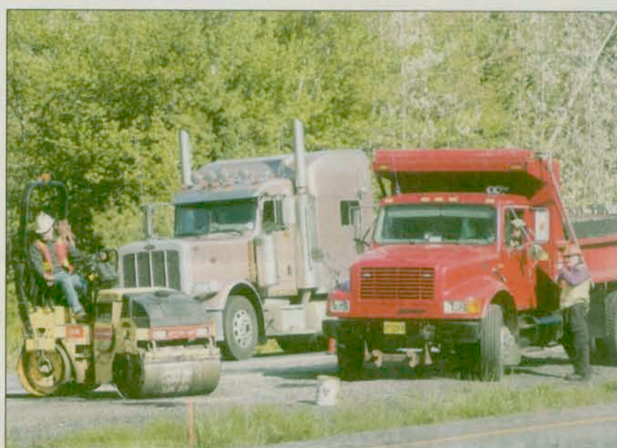
Road workers work on a section of the 102 just east of the airport May 2.
