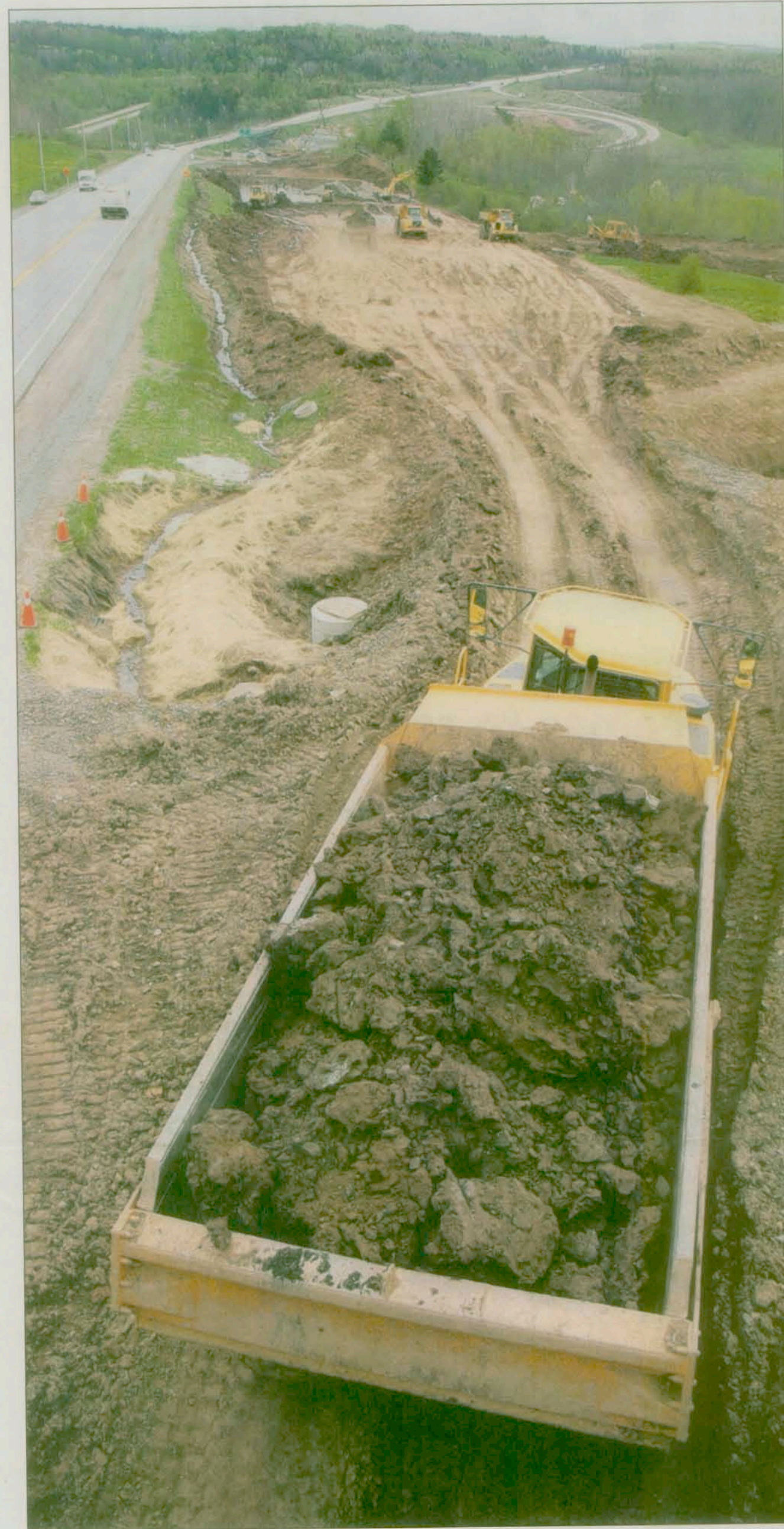
Road builders were busy working on the Highway 101 twinning project in this May photo.
