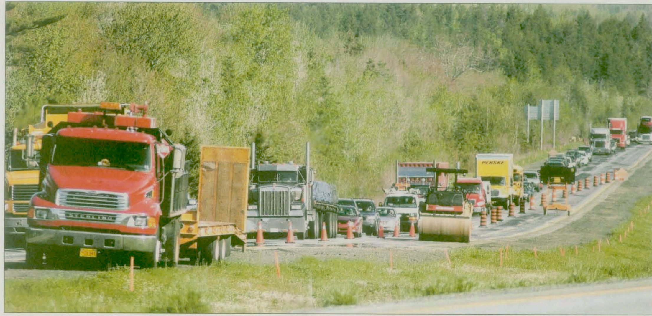
Work was ongoing on a section of Highway 102 near Exit 7 just past Halifax Stanfield International Airport June 2. It's important this time of year for motorists to be extra cautious and to start looking out for road builders on the job.
